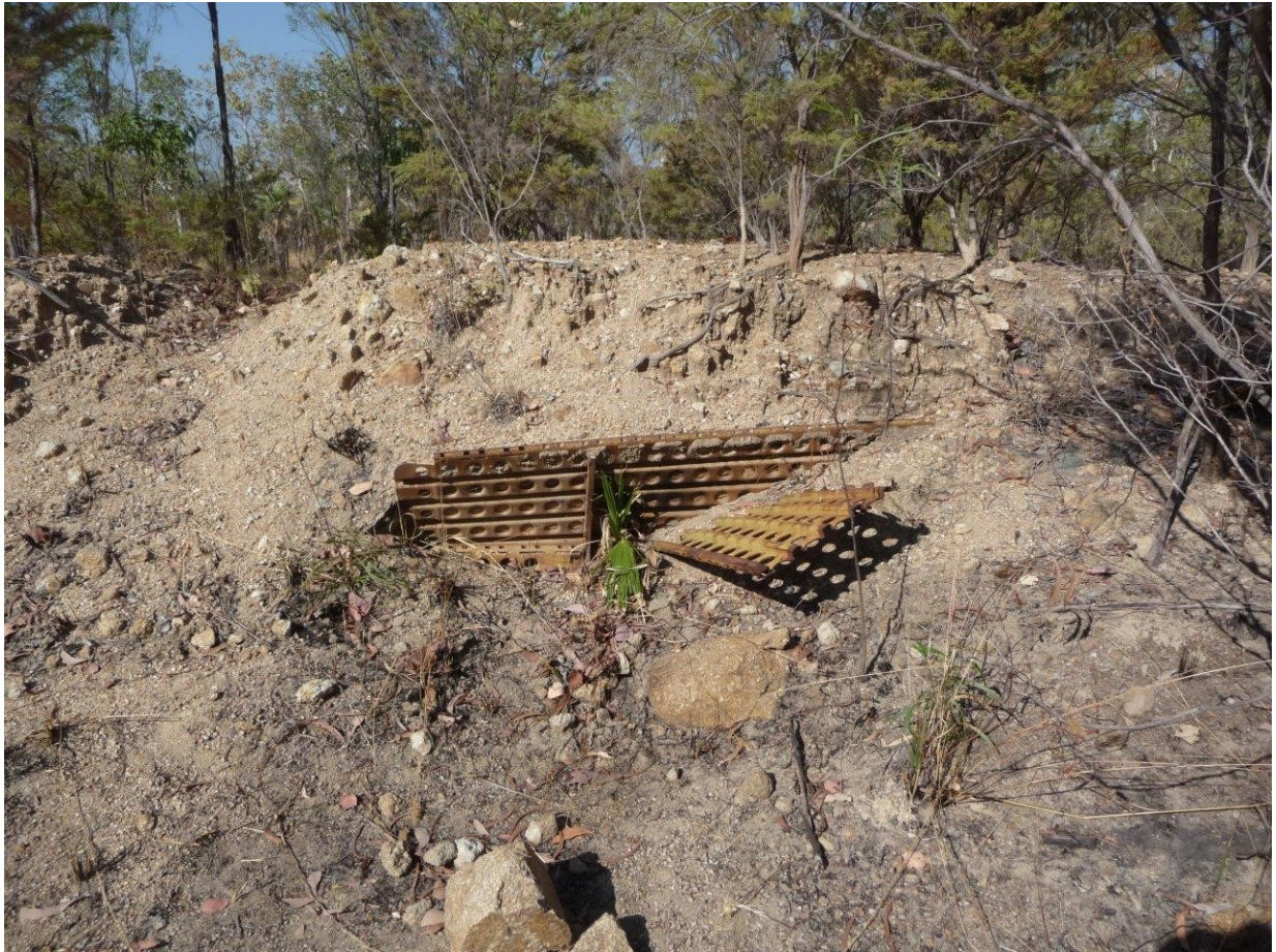
The wall is suffering from severe erosion, as are some portions of the taxiways. [Garry Shepherdson, 2015].
